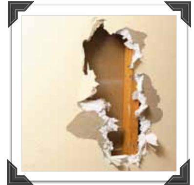
Front door swung open too quickly.
